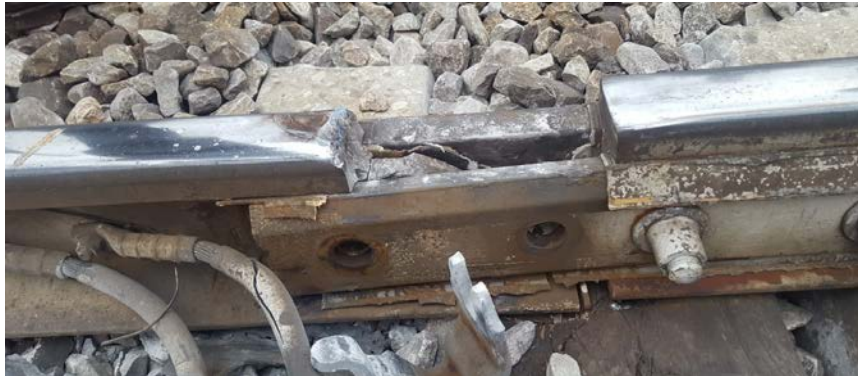
Figure 1. The joint broken in Pioltello on 25.01.2018. The train travels right to left. It can be seen that downstream portion of the IRJ is completely destroyed. The flown away portion of the railhead got stuck under a wheel causing the derailment of the train.
