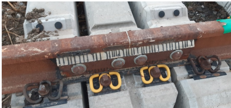
Figure 3. The IRJ currently used in Italy pictured before installation. A specifically widened sleepers was developed to (theoretically) better support the IRJ. Hollow sleepers to pass cables can be seen. Sleeper spacing is adjusted during installation but results to be non-standard with tamping difficulties.
